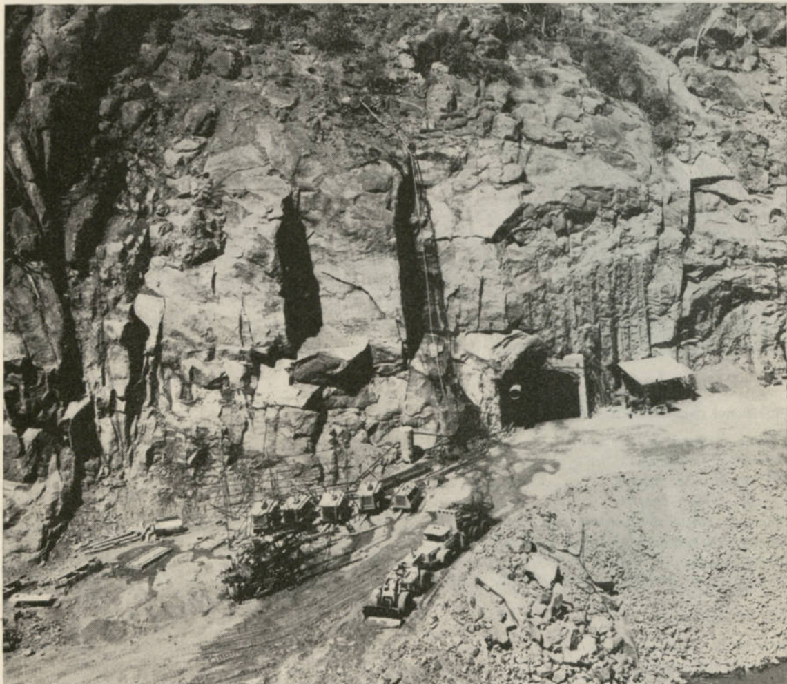
View of construction work in one of the tunnels of the Cabora Bassa Dam
